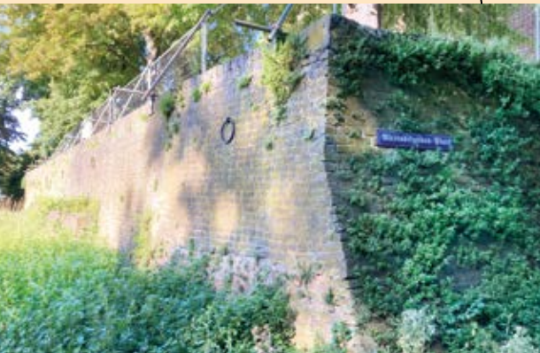
Quay wall below St. Gereon's Church. The long surface ran directly along the Rhine in the Middle Ages and served as a landing point for boats and barges. On the right of the picture, the angle of the wall leading eastwards is visible. The present form of the wall is mainly a result of the reconstruction of the church after the Second World War.
